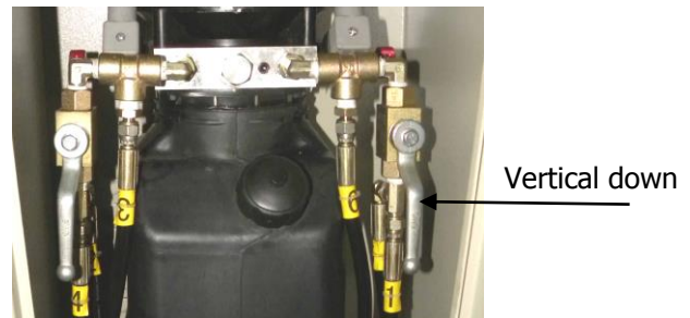
Oil Filling Position
